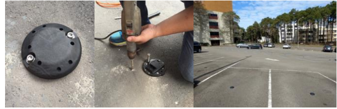
Fig. 10. NCTU parking application using NB-IoT.
